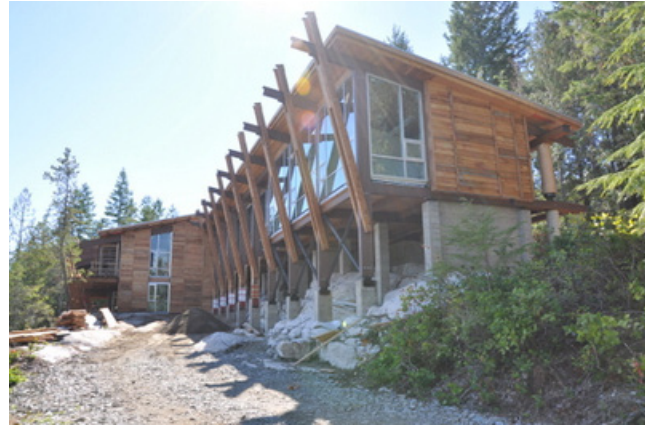
A new 15,000 sq. ft. office, health and multipurpose building on the Klahoose reserve nears completion
